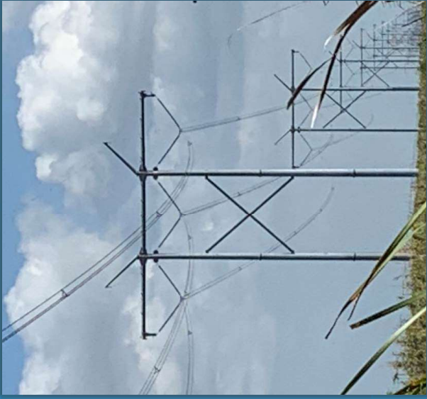
Transmission and substations
