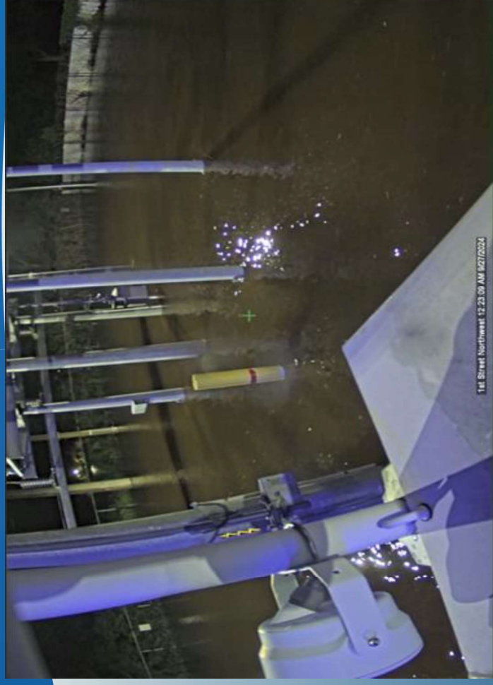
First Street Substation experienced storm surge during Hurricane Helene.
