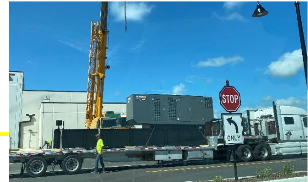
Generator in ICC 500 Enclosure
