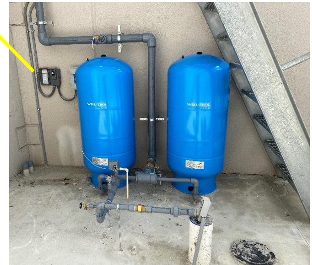
Inside ICC 500 built generator yard, back up well for sanitation water should main water supply from TCU be lost
