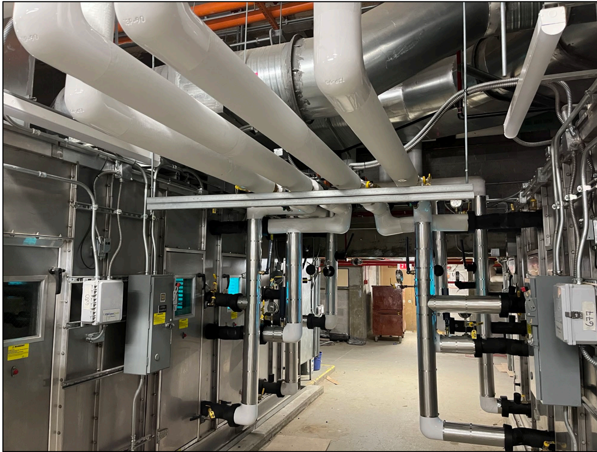
Capitol Tower New HVAC
